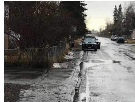
Parked car and remnants of plowed snow on a cracked, broken sidewalk.
